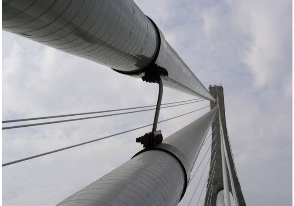
Figure 16.1.50 Cable Tie Type Damper System
