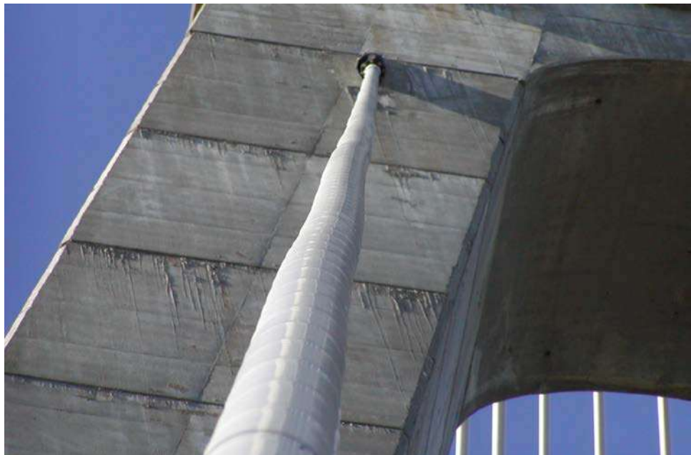
Figure 16.1.45 Bulging of Cable Sheathing
