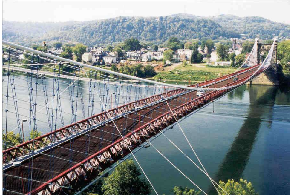
Figure 16.1.23 Cable Damping System - Wheeling Suspension Bridge (Photo Courtesy of Geoffrey H. Goldberg, 1999)
