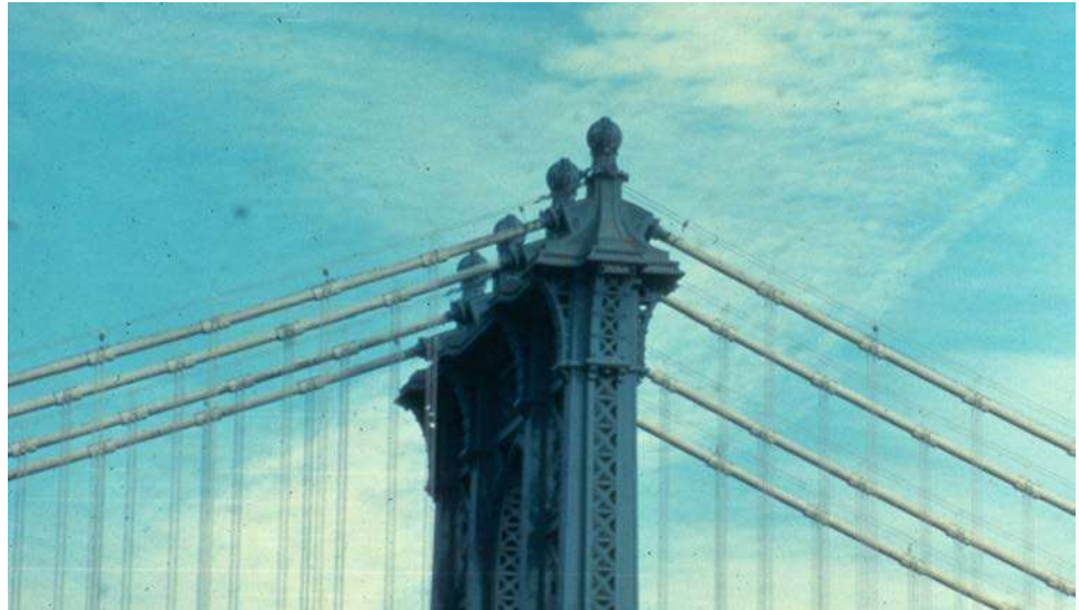
Figure 16.1.18 Cable Saddles for Manhattan Bridge, NYC (Main Span 1,480 ft) Suspender Cable Connections
