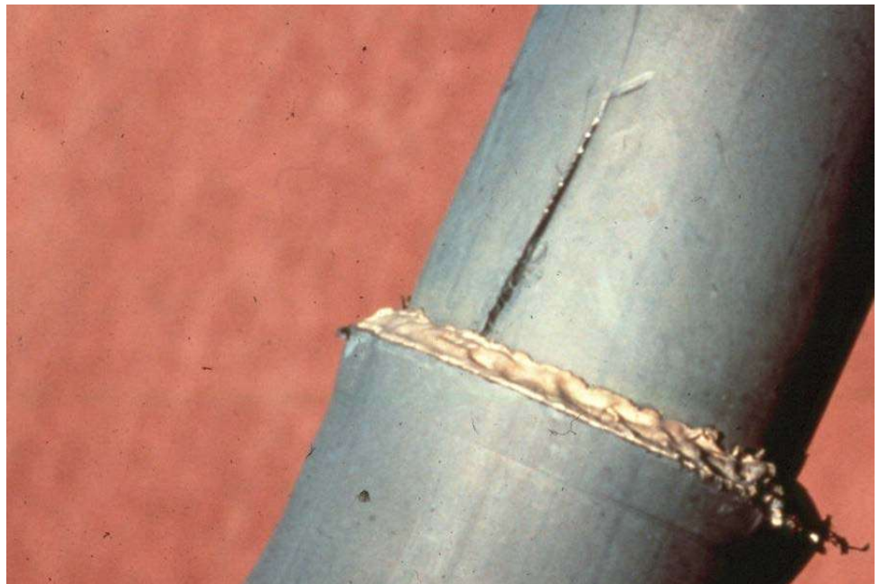
Figure 16.1.47 Splitting of Cable Sheathing
