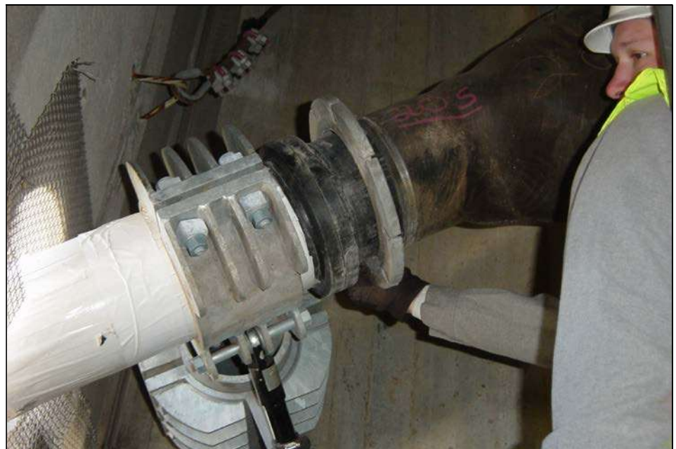
Figure 16.1.35 Damper on Cable-Stayed Bridge
