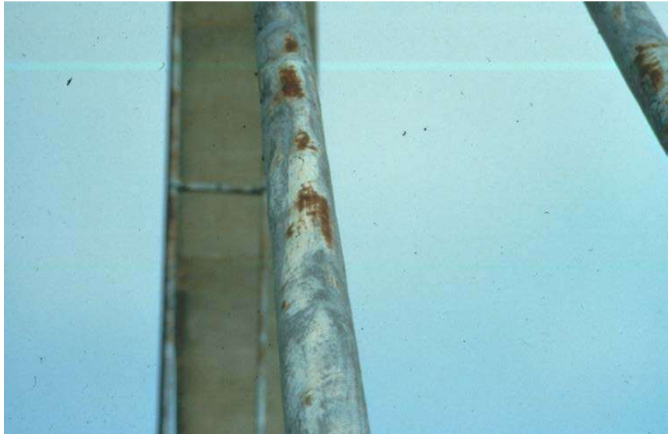
Figure 16.1.44 Corrosion of Steel Sheathing
