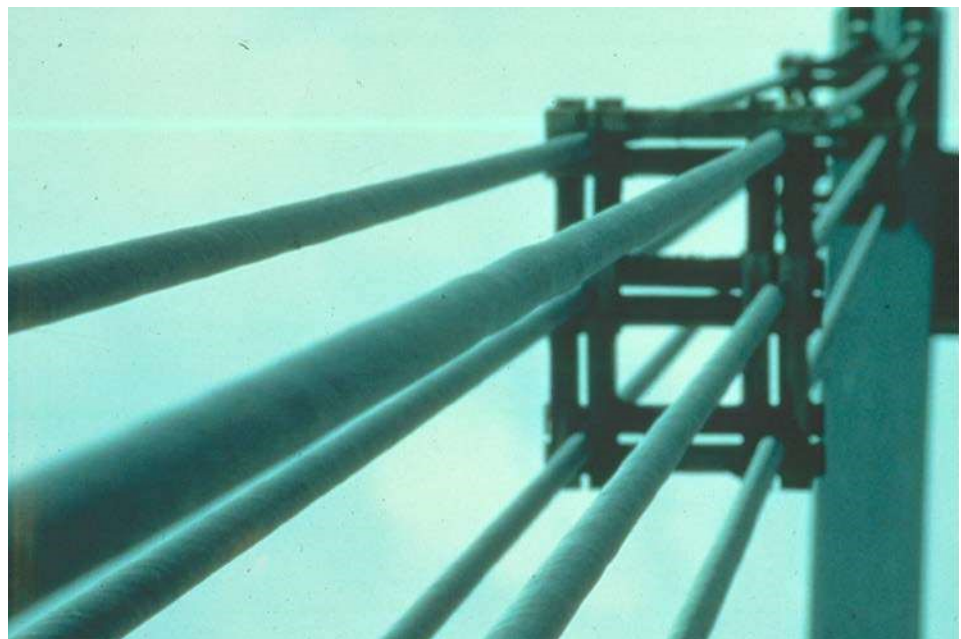
Figure 16.1.24 Cable Tie Damper System
