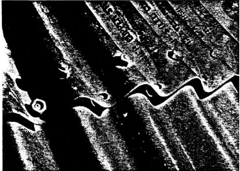
Figure 14.3.11 (Exhibit 69) Close-Up of Loose and Missing Bolts at a Cusped Seam; Loose Fasteners are Usually Detected by Tapping the Nuts with a Hammer
