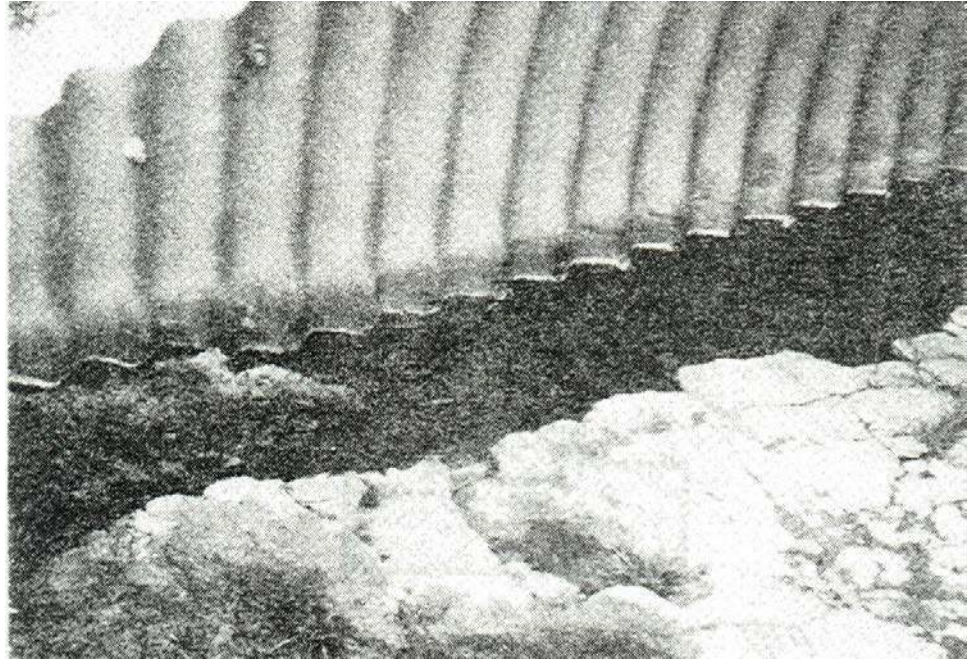
Figure 14.3.21 (Exhibit 79) Erosion Damage to Concrete Invert
