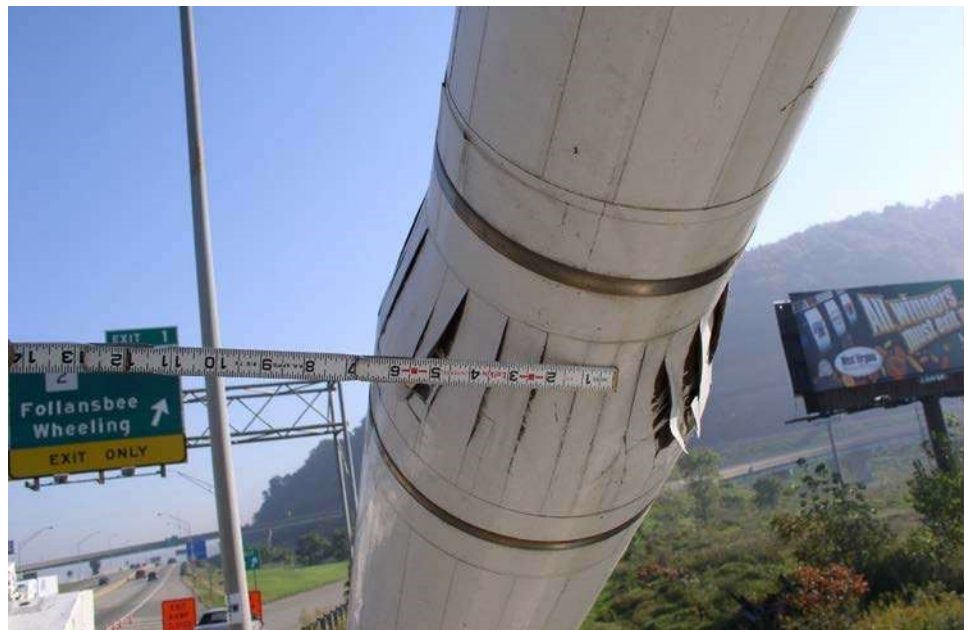
Figure 16.1.43 Deformed Cable Wrapping
