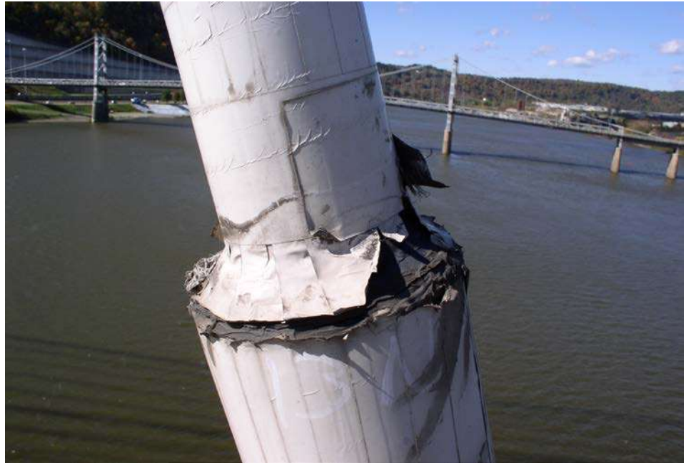
Figure 16.1.38 Tape and Rubber Seal Torn Around Cable Allowing Water Penetration into Top of Sheath
