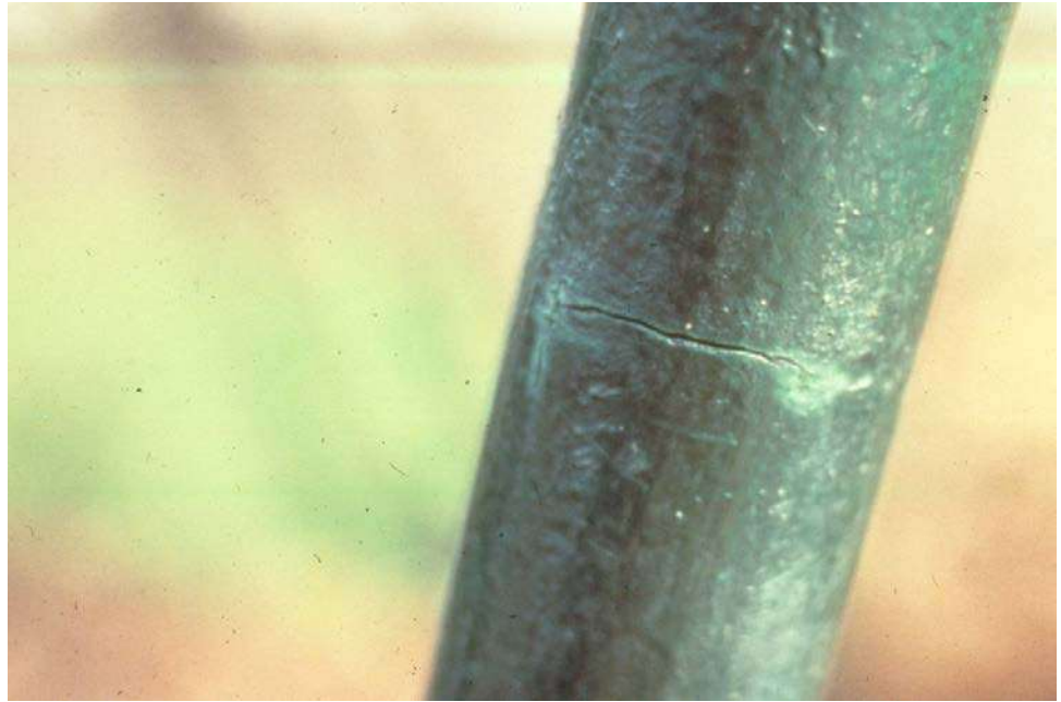
Figure 16.1.46 Cracking of Cable Sheathing
